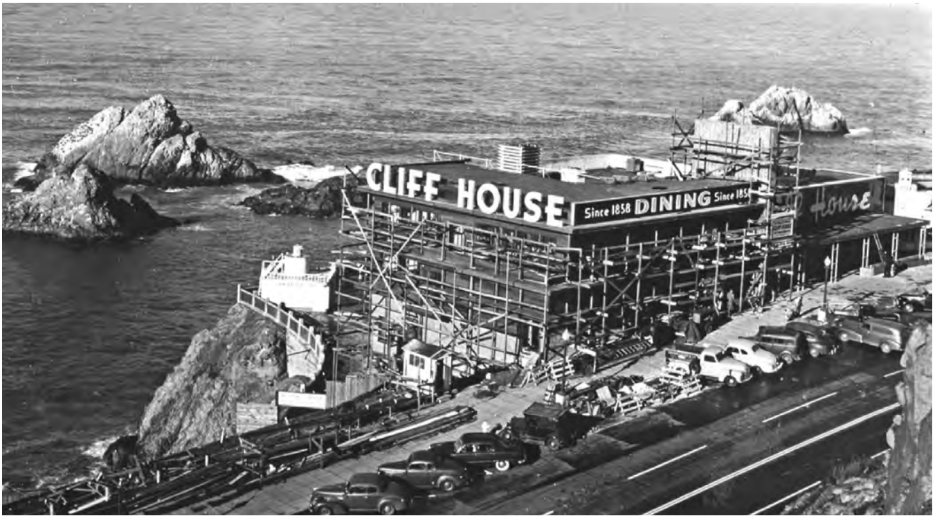
Third Cliff House undergoing remodeling, circa 1950. Image from Cliff House Project, courtesy of Gary Stark.
